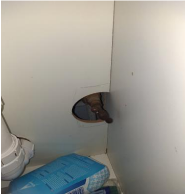
Mains Isolation Valve
