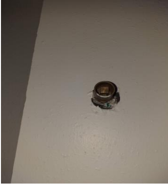
Mains Isolation Valve
