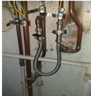
Filling Loop Connected at Boiler
