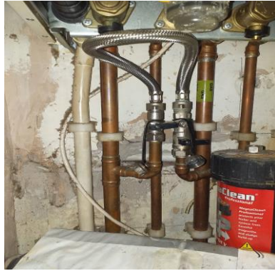
Filling loop connected at boiler
